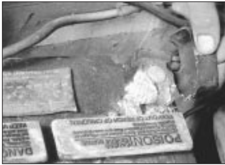
6.6a Battery terminal corrosion usually appears as light, fluffy powder
