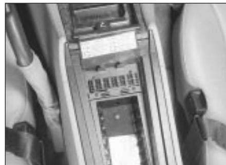
3.1c A third fusebox is located in the centre console glove box
